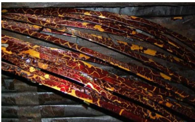
Fig. 5: LV winding of a 110 MVA GSU transformer, DP mean average < 200
