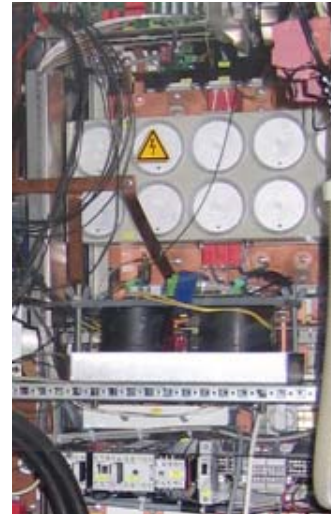
Fig. 13: Power stack of the voltage sourced converter
