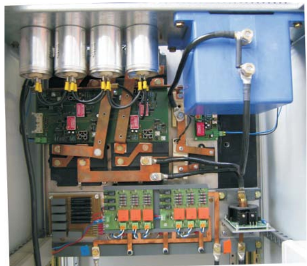
Fig. 14: Power stack of the current sourced converter
