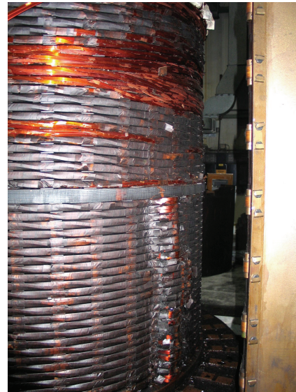
Fig. 12: Radial buckling of LV winding
