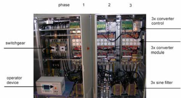
Fig. 7: H-Bridge Inverter (300 kVA) and HMI
